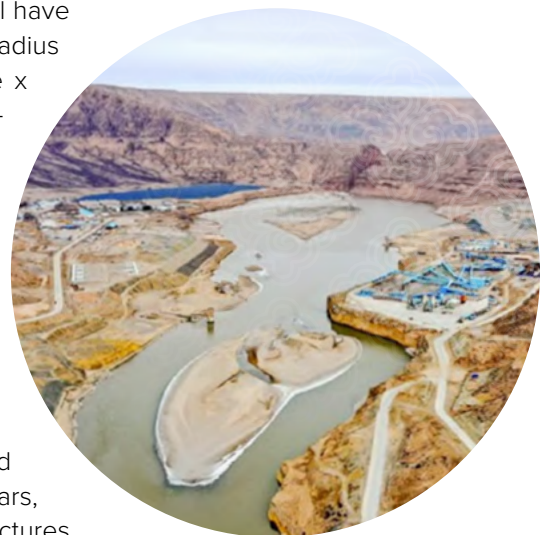
Yangqu dam under construction. Source: Radio Free Asia, 12 April 2024, via citizen journalist.
