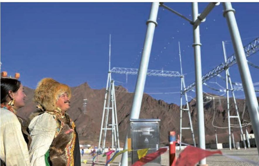
This image from the Chinese state media shows the launch of the electricity grid between the Tibet Autonomous Region and Sichuan on November 20, 2014. The rapid dam-building in Tibet is intended to produce energy in hydro-electric power stations to be conveyed along high-voltage transmission lines for China's expanding urban centers far from Tibet.
